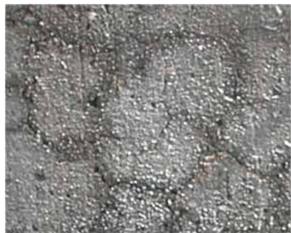
Fig. 4.6.5.2: Crack pattern as seen on the concrete surface. The picture covers an area of about 400 mm x 400 mm and was taken near the most severely damaged concrete close to water level.
