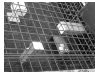
Block 1 "voids" 6, 11, 12 and steel plate cast in with semi-spherical "voids" on upper side.
