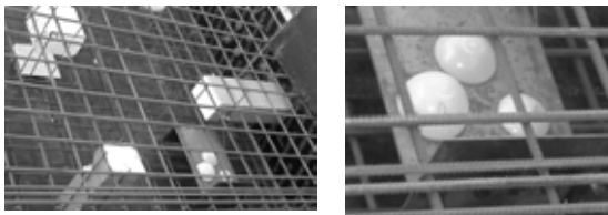
Fig. A.4.17: The steel plate cast in Block 1 (260 mm from the underside). In the left-hand figure the artificial voids can be seen on top of the plate. The steel plate is 8 mm thick. Some semi-spheres made of plastic have been glued to the top of the plate to represent voids inside the concrete adjacent to the (back of) plate. Scans were made along the underside of the slab in line with the two voids nearest the edge (closest to the camera in the photo above).
