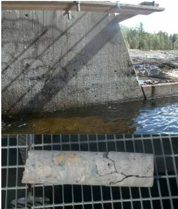
Fig. 2.5.1: A dam pillar in the north of Sweden. The concrete is suffering from freezing damage as well as ASR. Tests were made to find out how deep the cracks extended from the surface.
