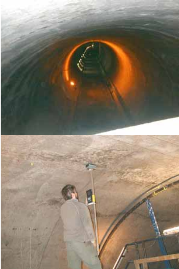
Fig. 2.2.1: Tunnel with in-situ cast concrete liner (nominal thickness 600 mm). The thickness of the concrete is being measured using ultrasonic pulse echo.
