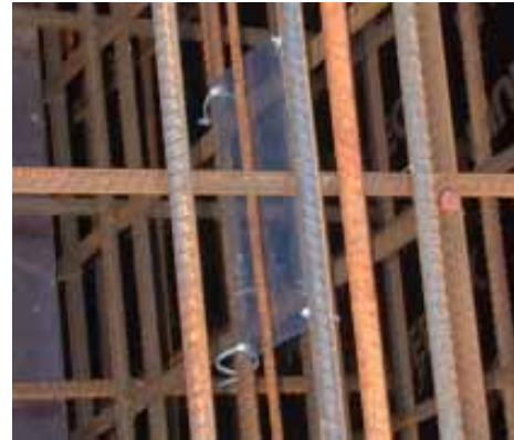
Fig. A.1.4: South face of Block 1 with thin plastic sheet securely fixed to the reinforcing. Notice that a thin bar has been fixed behind the sheet to prevent movement or bending.
