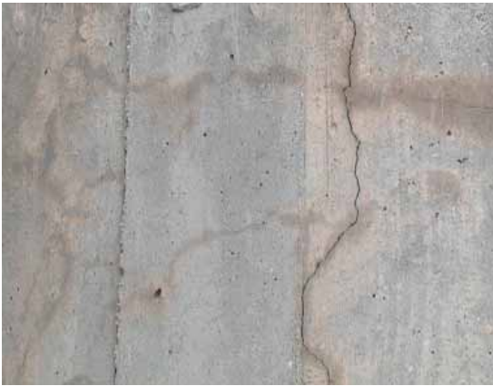
Fig. 4.6.5.6: Bridge column with map cracking (shady and moist-like edges suggestive of ASR.) Larger vertical surface open cracks appear at regular intervals around the column, as well as map cracking.
