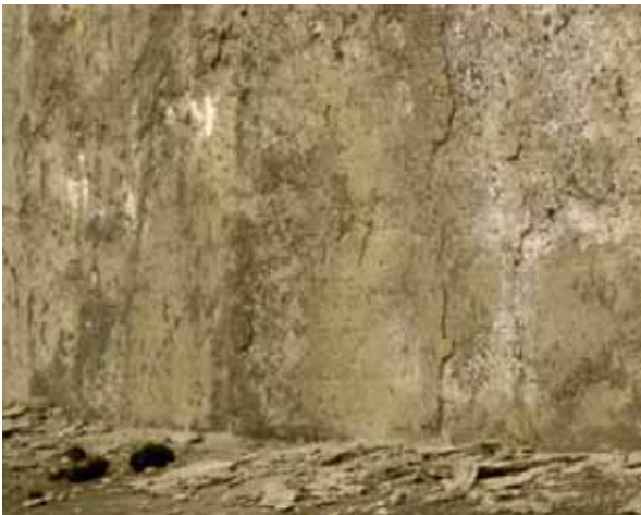
Fig. 4.6.5.13: There were obvious signs of frost scaling also.
