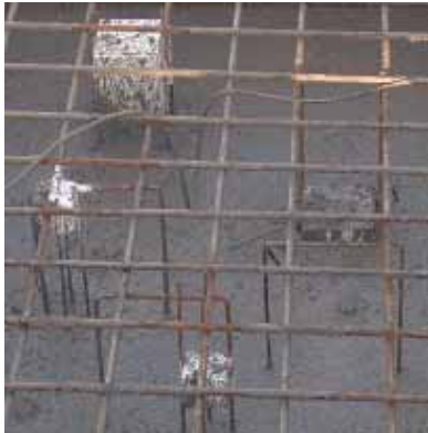
Fig. A.1.3: Block 1 during casting with square voids fixed in place. In the upper part of the picture we see two 200 mm cubes at 220 mm and 490 mm depth respectively.
