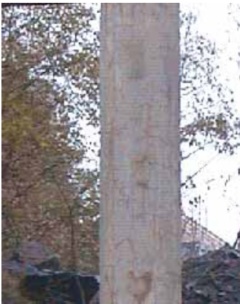
Fig. 4.6.5.7: View of the column. The cracking is obvious along the whole length of the column, but most clearly on the side, which is exposed to the prevailing weather (higher moisture levels).
